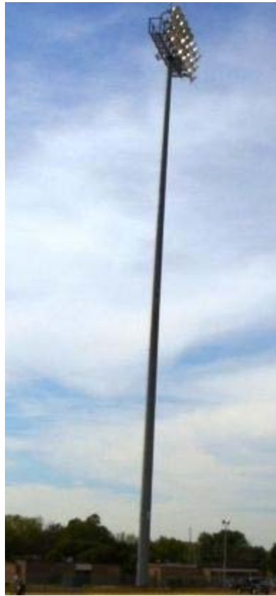
Upright Stadium Light Pole
