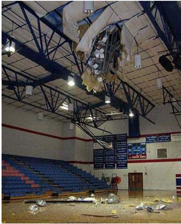
Stadium Light Pole Fallen Through Gymnasium Roof
