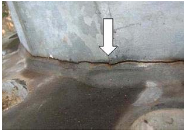
Close-up – Crack Near Weld that Joins the Pole to its Base Plate
