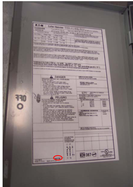
Figure 3. The red circle indicates where the date code is located on the pub inside the case of the switch
