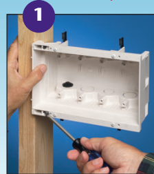
1 Mount box to stud. Use tabs for proper positioning of box for 1/2" wall finish. See Photo A.
